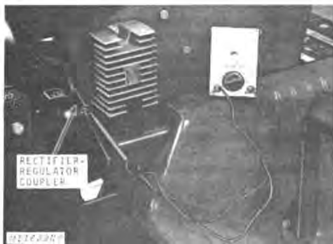
Fig. 4-Checking AC Voltage Output
